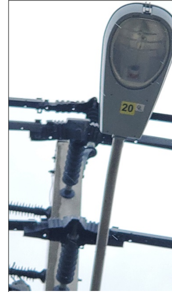
Figure 1 - Photo of an existing HPS luminaire on Estero Boulevard
